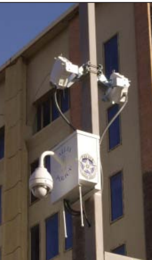
Video system components used outdoors by the city of Dallas are mounted inside protective weather-resistant enclosures.
